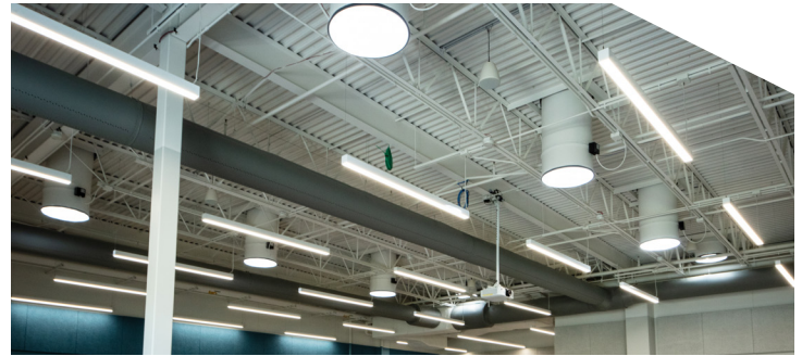
Piper Elementary School / Kansas City, KS Solatube
