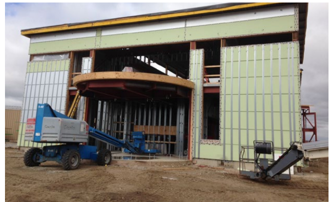
6. After Genwall and windows have been installed, the building has a complete air barrier and is weathered in.
