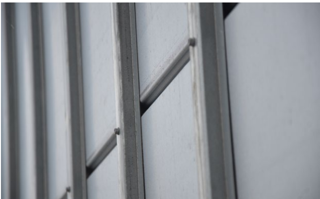
5. Genwall hat channels are installed. Buildings can easily be re-skinned without disturbing the interior wall system.
